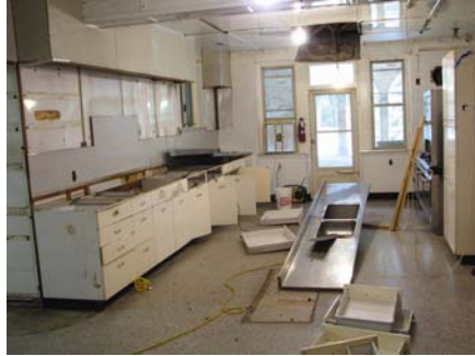
Demolition of the kitchen began with the removal of the center serving islands, followed by the sinks and cabinets. Removal of the linoleum walls and metal ceiling followed.
