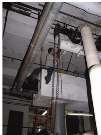
Frank sits on the furnace as he works on the conduit to the kitchen.
