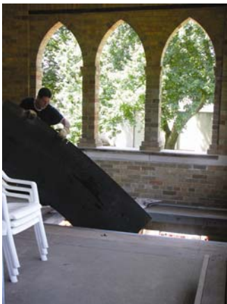
A workman carries one of the steel kitchen wall panels to the cloister coffin hatch (yes, we have a coffin hatch!) for scrapping.
